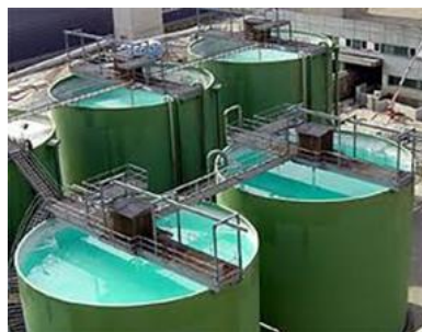
Figure F.23: Brine purification plant lxix
